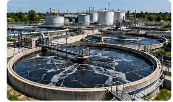
Wastewater & Effluent Treatment
